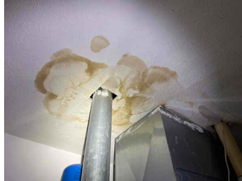
Right Utility Room, Ceiling Stains, Dry When Tested
