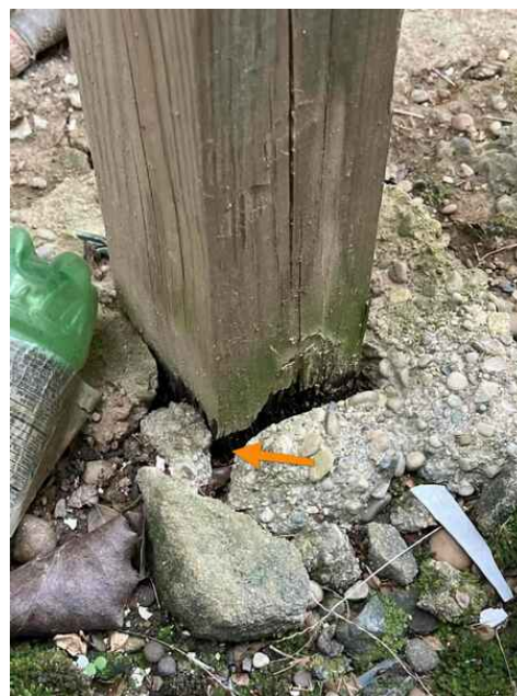
Side Steps, Rotting Post - Example
