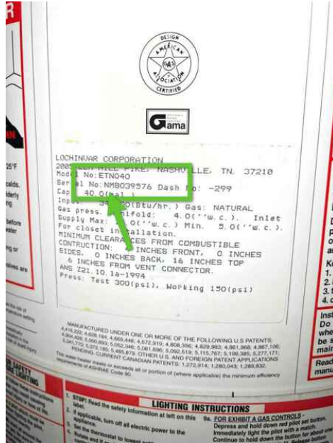
Left Side Hot Water Tank Age, 1996
