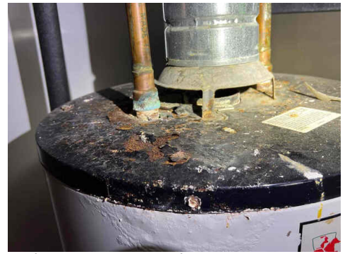
Right Hot Water Tank, Corrosion
