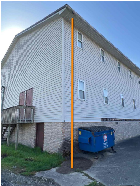
Left Side of Building, Downspout Missing
