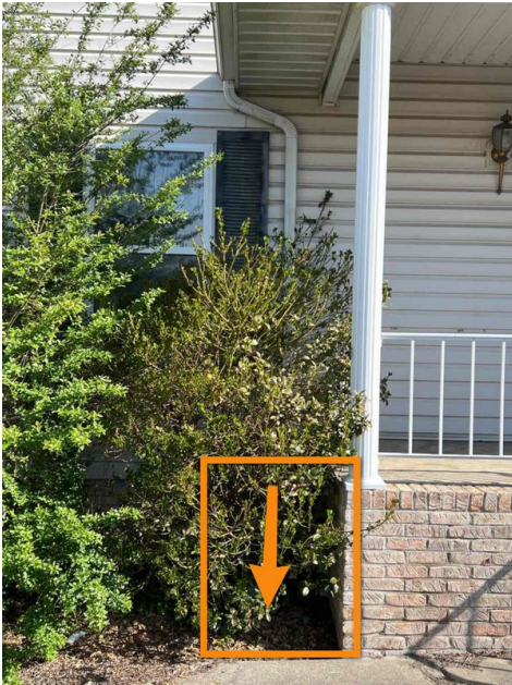
Front Porch, Downspout Drains on Ground
