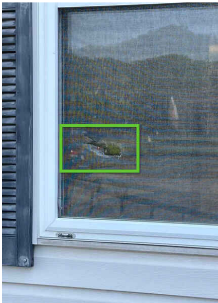
Front of Building, Both Windows Have Torn Screens
