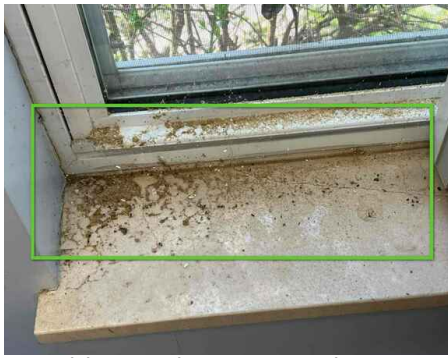
Lobby Window, Potential WDI
