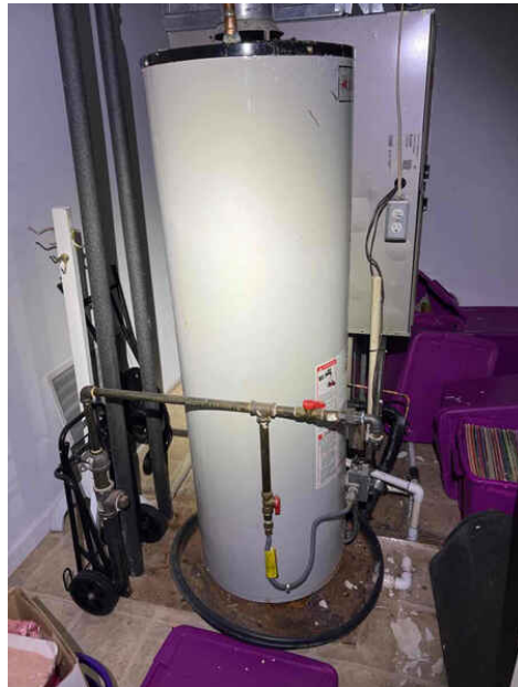
Right Side Hot Water Tank
