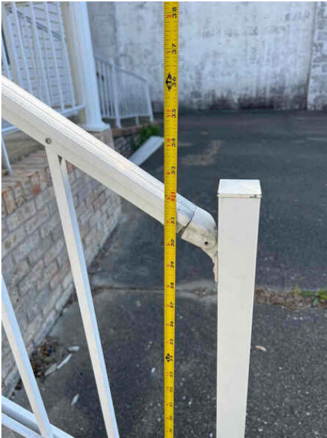
Front Porch Railing Height, Recommend 42"
