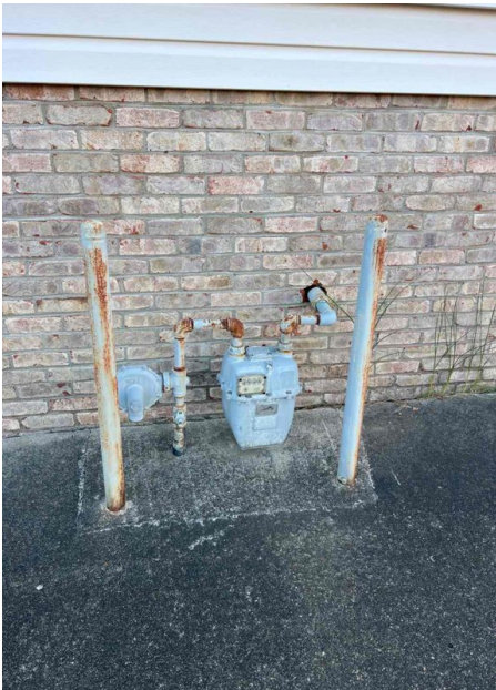
Main Gas Shutoff, Left Side of Building
