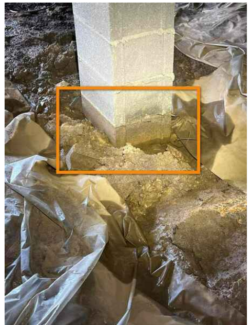
Example - Crawlspace Floor Support Pillar, Standing in Water
