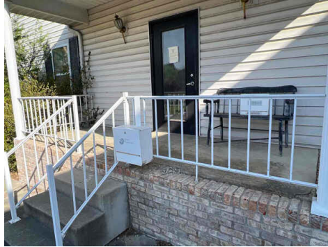
Front Porch Railing Height, Recommend 42"
