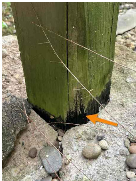
Side Steps, Rotting Post - Example
