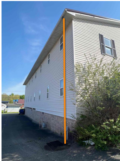
Left Side of Building, Downspout Missing
