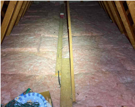
Attic Insulation Example
