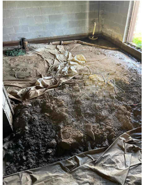
Crawlspace, Muddy Conditions, High Moisture
