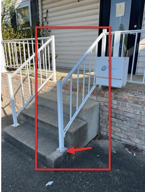
Front Steps, Handrail Not Secure
