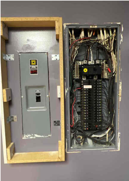
Main Electrical Panels
