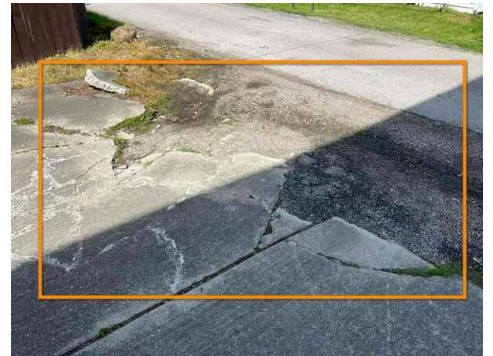
Parking Lot Deterioration
