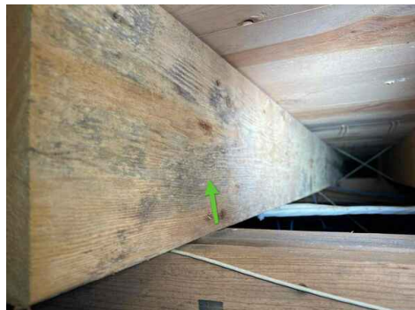
Potential Mold - Crawlspace Example
