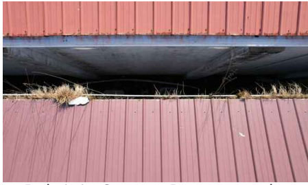
Debris in Gutters, Recommend Cleaning
