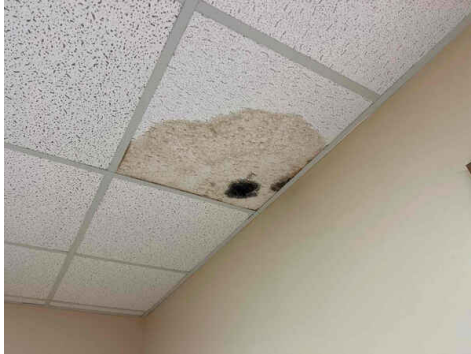
Center Lab, Ceiling Stain (Mold), Dry When Tested
