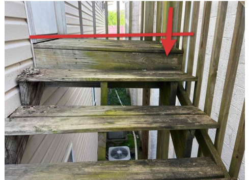
Side Steps, Nearing End of Life
