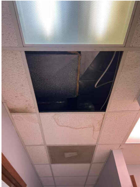
Left Hallway, Ceiling Tile Missing (Below Left Furnace)
