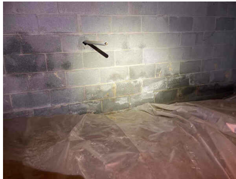
Example of Moisture Thru Block, From Downspouts and Negative Grading
