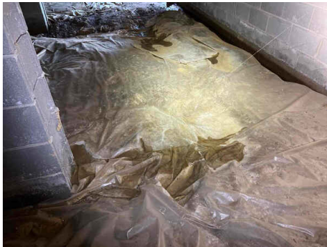
Crawlspace - Example of Standing Water
