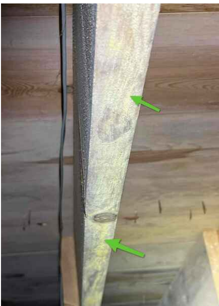
Potential Mold - Crawlspace Example
