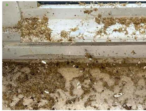
Lobby Window, Potential WDI
