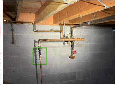
Main Water Shutoff Valve, Crawlspace
