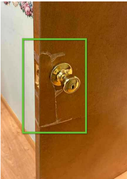
Dr Office Door Damage
