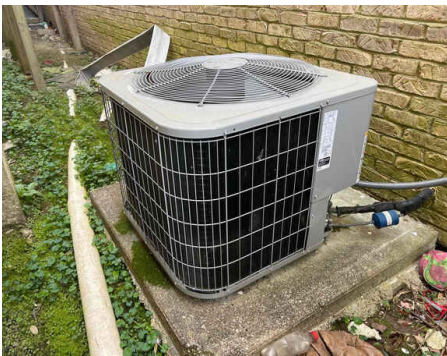
#2 Air Conditioning Unit - Right Unit
