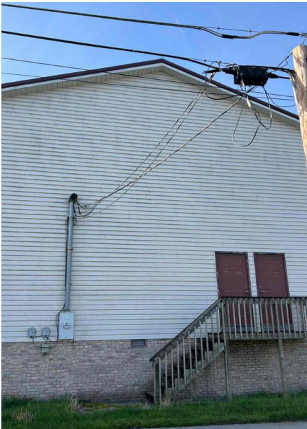
Power Service Entrance Cables
