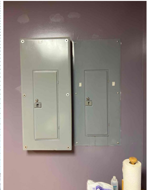
Main Electrical Panels
