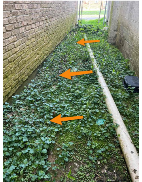
Negative Grading Between Buildings
