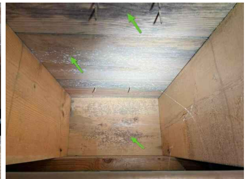
Potential Mold - Crawlspace Example
