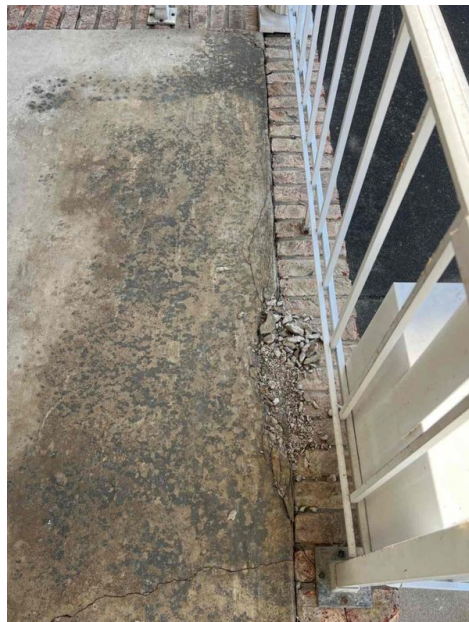
Front Porch, Concrete Deterioration
