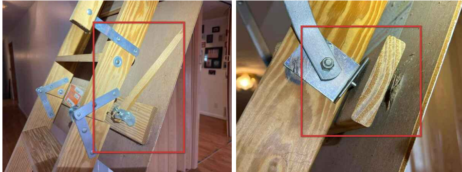
Attic Stairs Damaged, Use With Caution Attic Stairs Damaged, Use With Caution
