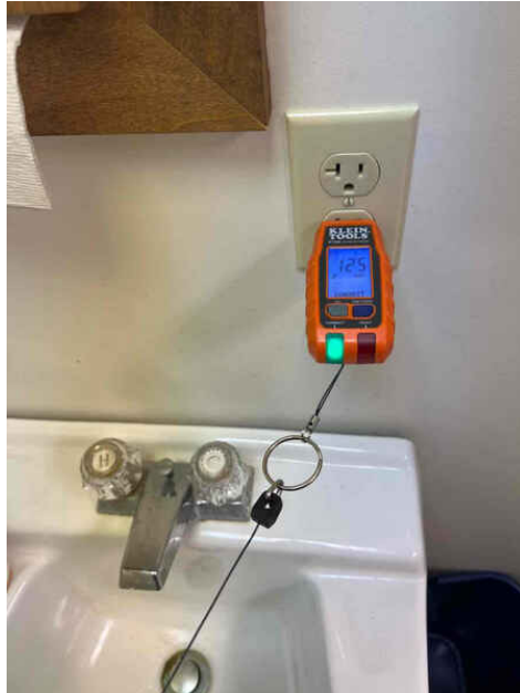
Example Bathroom - GFCI Protection Missing - All Bathrooms
