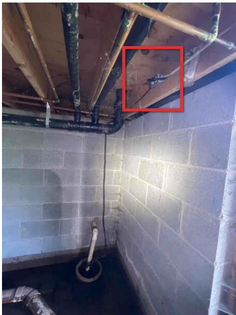
Crawlspace, GFCI Protection Missing
