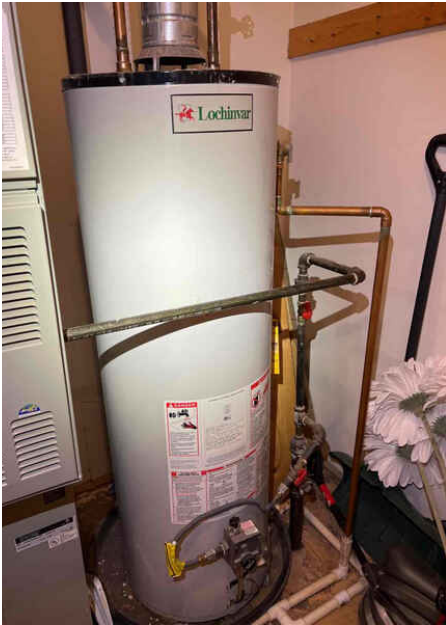
Left Side Hot Water Tank
