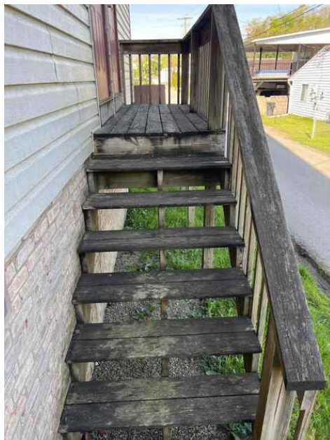
Rear Steps, Nearing End of Life
