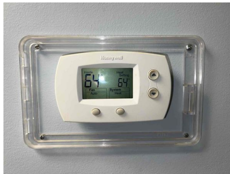
Right Hallway, Thermostat
