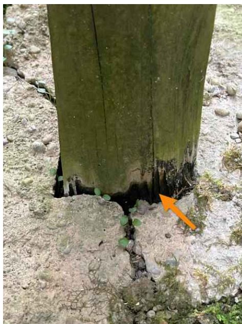
Side Steps, Rotting Post - Example
