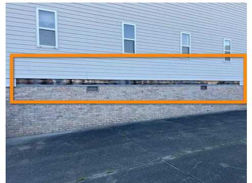
Left Side of Building, Missing Siding
