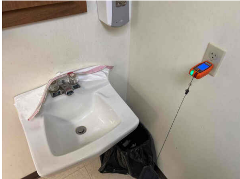
Example Bathroom - GFCI Protection Missing - All Bathrooms
