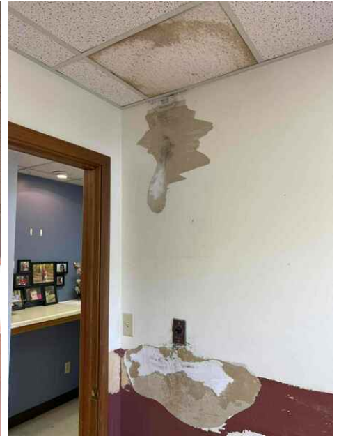
Below Left Furnace, Ceiling and Wall Damage from Water
