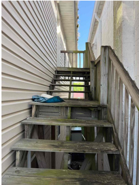
Side Steps, Nearing End of Life
