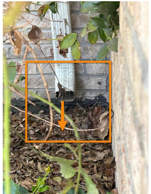
Front Porch, Downspout Drains on Ground
