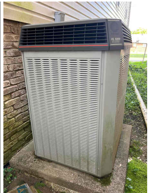
#1 Air Conditioning Unit - Left Unit
