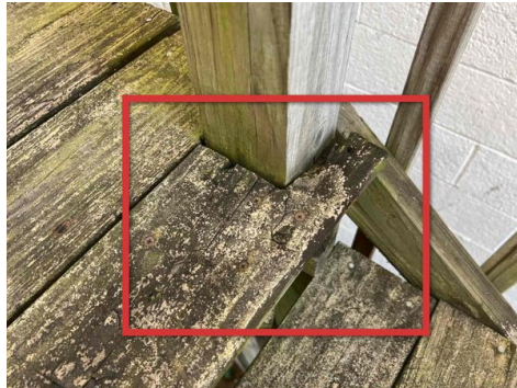
Side Steps, Nearing End of Life
