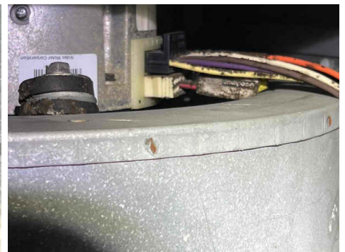
Attic, 2nd Floor Furnace, Mold
