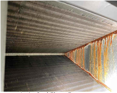
Attic, 2nd Floor Furnace
