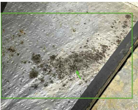
Attic, 2nd Floor Furnace, Mold
