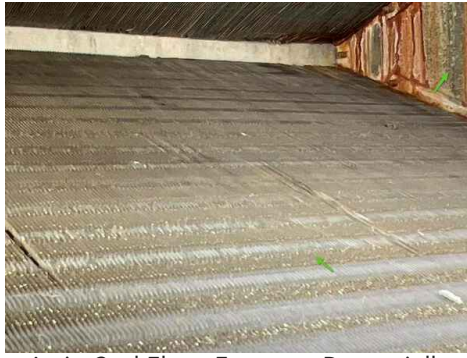
Attic, 2nd Floor Furnace, Potentially Mold
